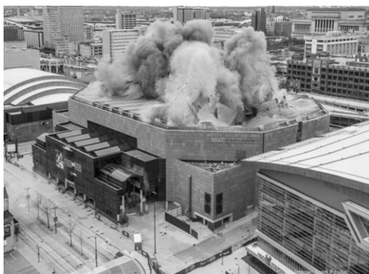
Fig. 5. Fot. Scott Paulus: Bradley Center demolition Ryc. 5. Fot. Scott Paulus, Źródło: www.bizjournals.com/milwaukee/news/2019/02/06/see-the-latest-in-demolition-of-the-bradley-center.html
